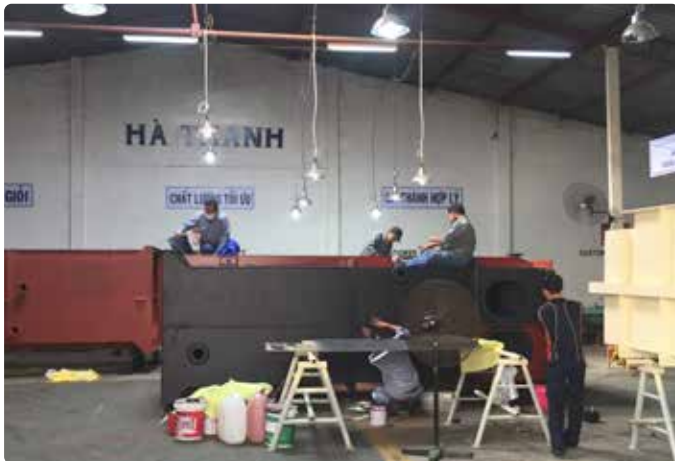
Both face tank Rubber lining at HT Shop
