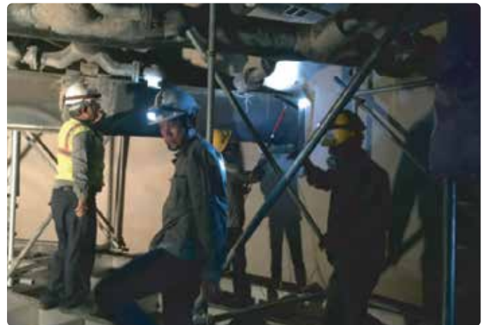
FGD side shell check
