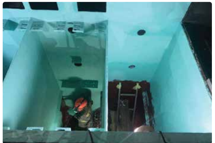
Pickling Resin Tank
