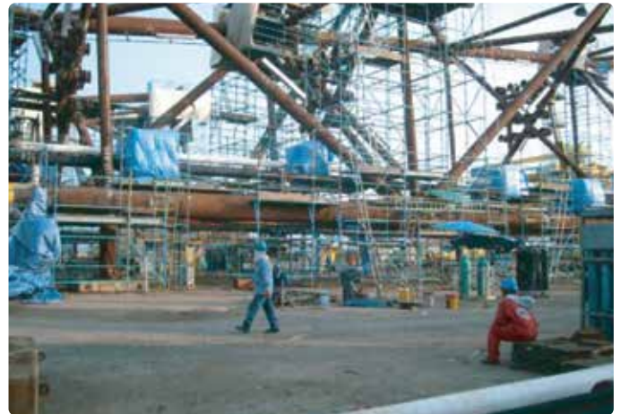
Riser clamps assemblies with Neoprene lining
