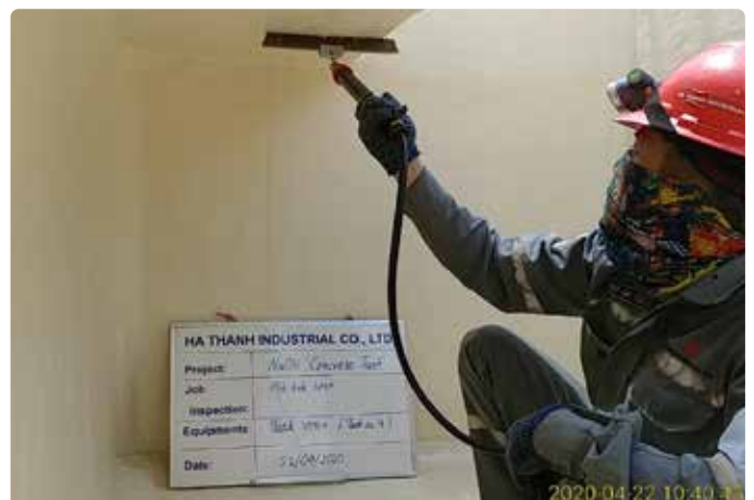
Pinhole check quality
